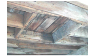
The storage areas were linked by cross passages, stairways, and four internal lifts transporting goods through hatches between the different levels (left).
